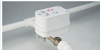
Photo 11. Manual control of the ball valve
